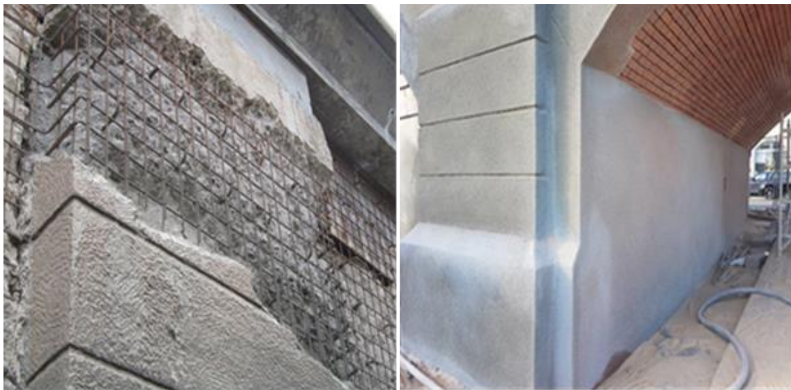
Figure 10: Damaged rustication of the support before and after repair. Visible brick vault repair
