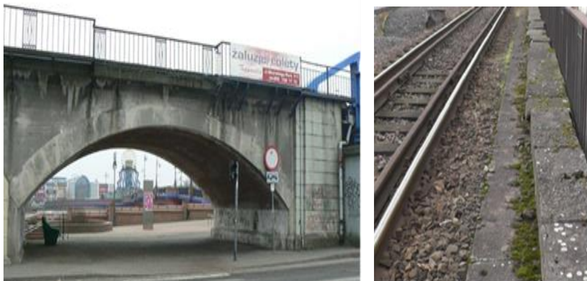
Figure 3: View of a typical open brick-concrete bay and the original railway track with a cornice and steel railing
