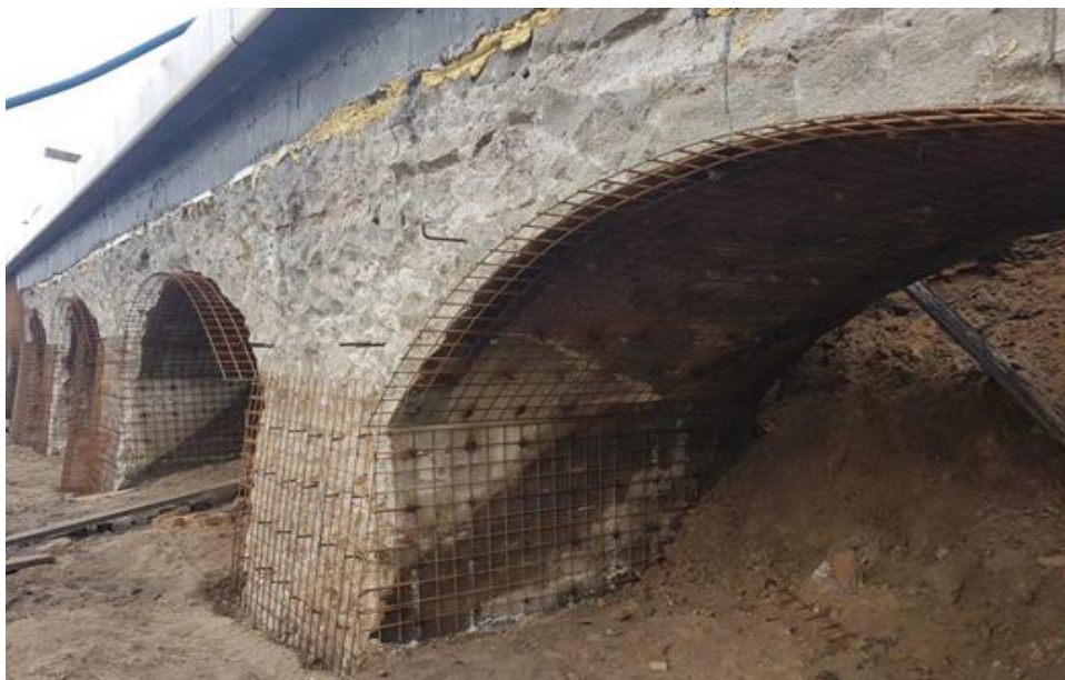
Figure 6: View of the spans after removal of old concrete and mounting of reinforcing mesh
