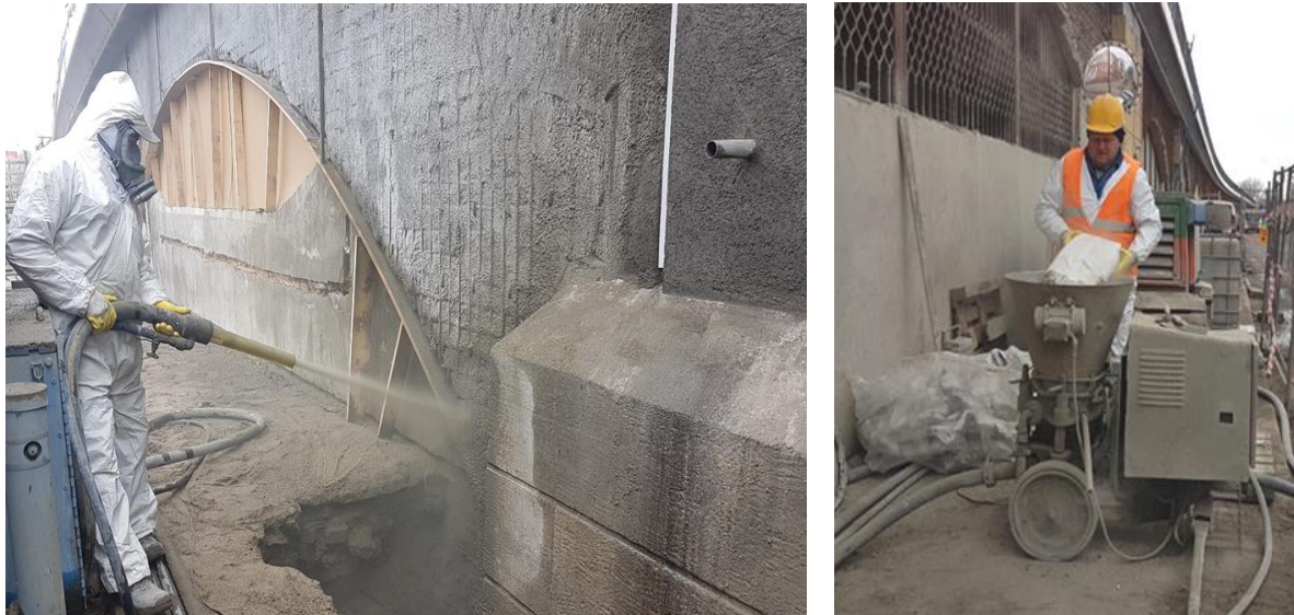
Figure 7: Spraying the second layer of shotcrete (reinforcement cover 3 cm). In the right the ALIVA 246 machine
