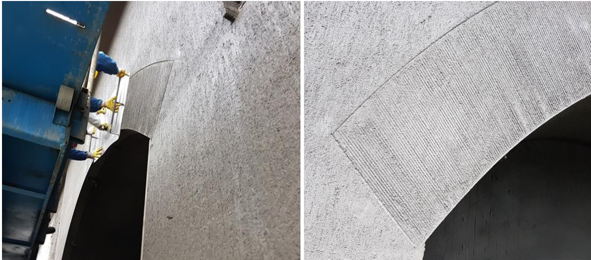
Figure 9: Grooving the lower part of the arch - steel sheath with vertical cuts and manual line profiling
