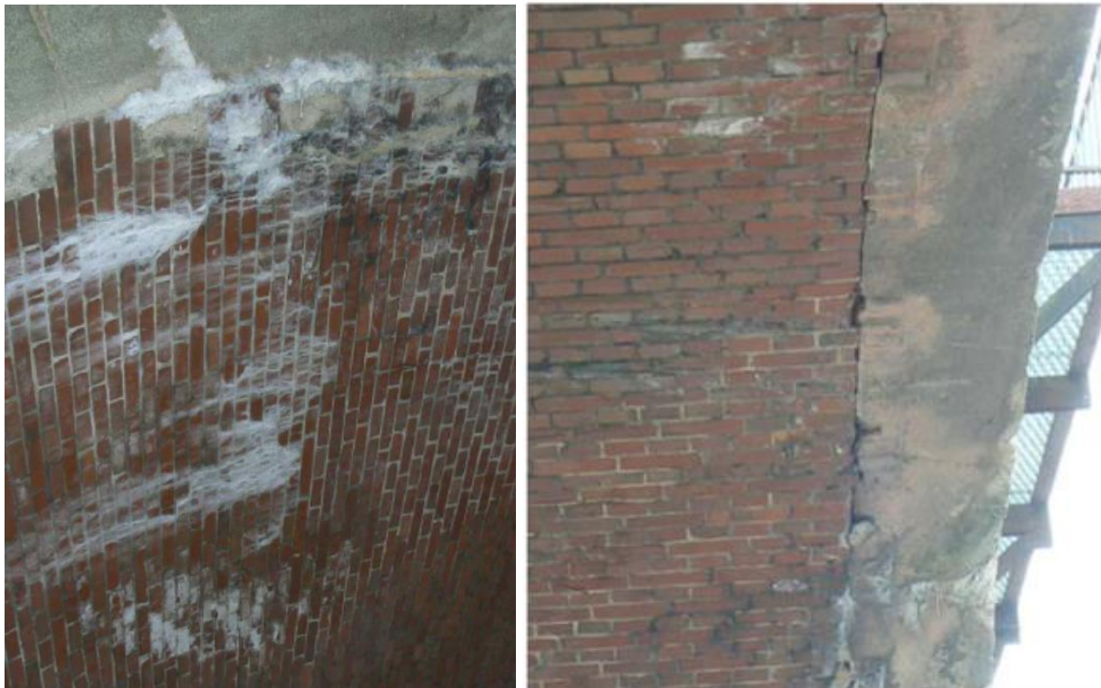
Figure 5: Brick vault and concrete arch end (bottom view). Leaks, efflorescence, defects in bricks and concrete, cracks on a concrete arch
