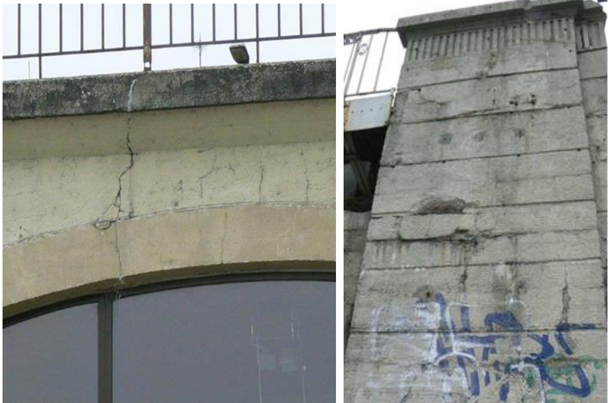
Figure 4: Cracks in the brick and concrete arch and supporting elements
