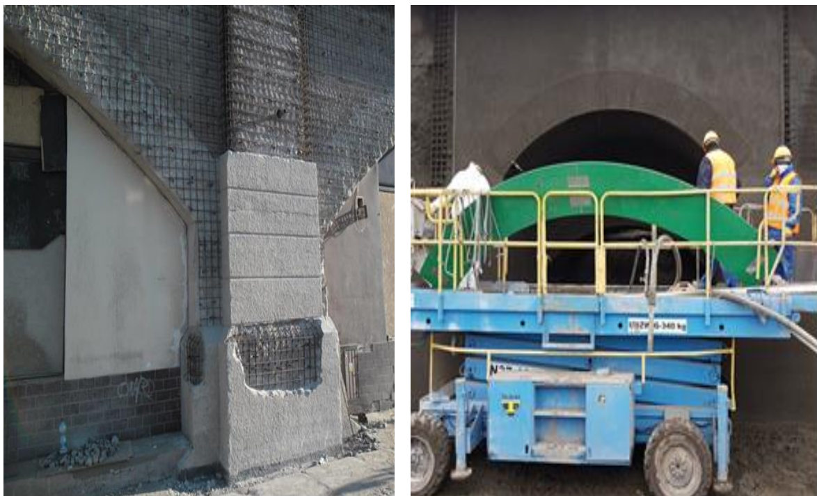
Figure 8: Preparation and reinforcement of the surface in the area of support of the flyover arch with damaged rustication. Visible green template used to imprint the arch in the fresh concrete
