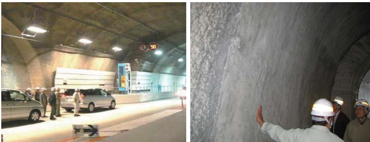
Figure 10: ECC application at emergency parking zones (left) and surface finish of ECC coating after completion (right).
