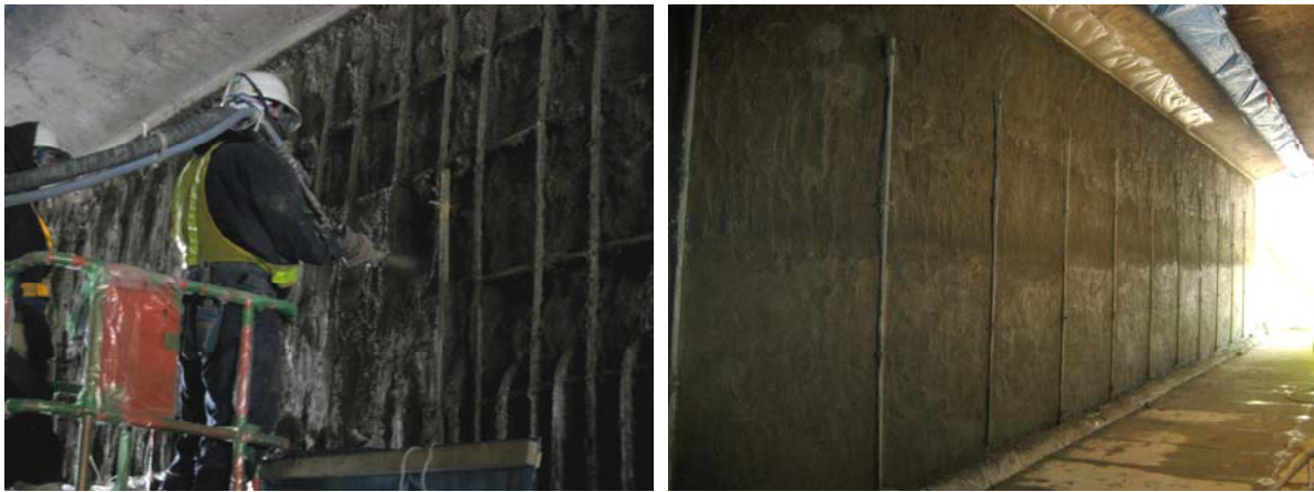
Figure 9: Replacement of chloride-infested concrete with ECC (left) and prefinished surface after replacement (right).
